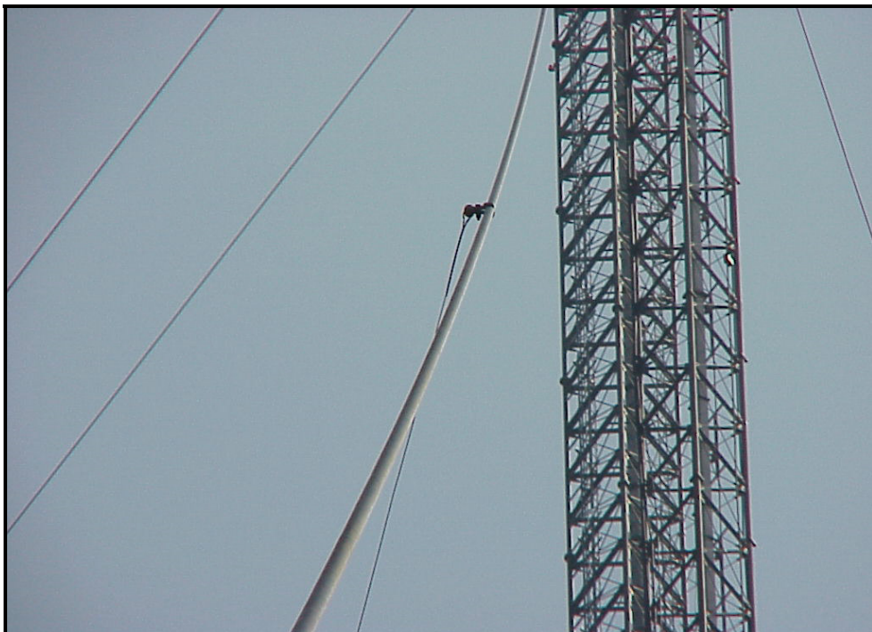
AR SNUBBER - Installed
