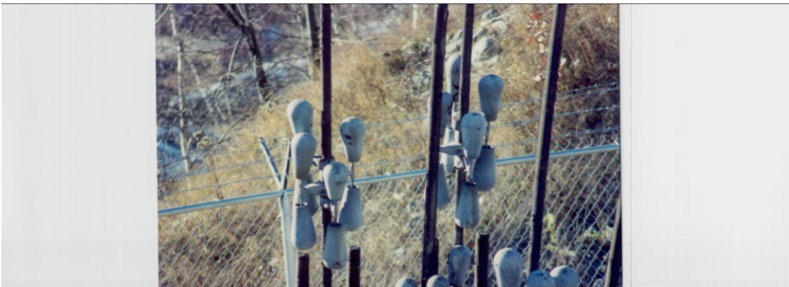
Photo #1 Stockbridge dampers attached to TV tower guy cables
