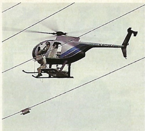
3. Windampers are spaced one-third of the span length from each tower. Two devices are needed per span-phase (above)
