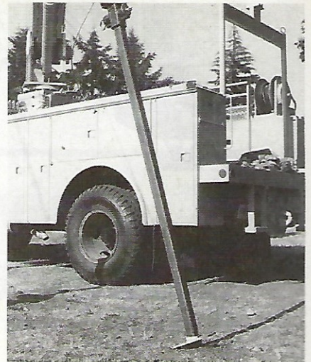
1. Anchor being driven by truck-mounted installer. Correct anchor size and depth ensure trouble-free guying
