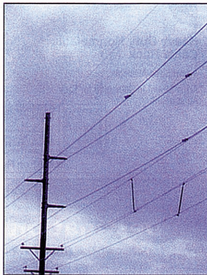
Fig. 1. Transmission and distribution lines on a single set of poles.
